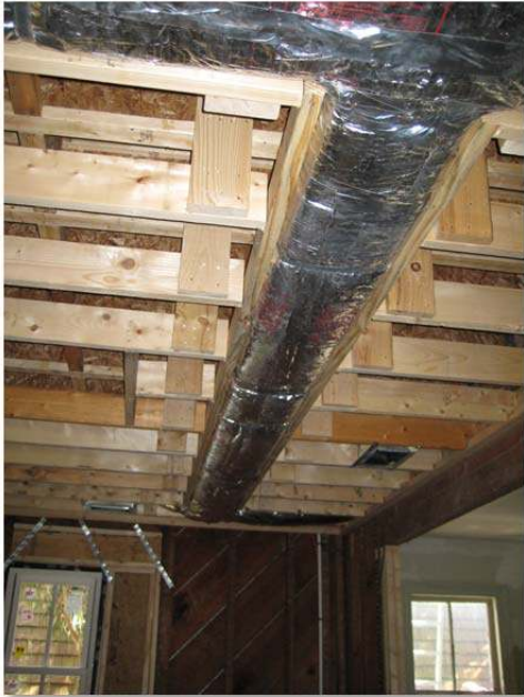
Duct run in "Chase" in kitchen Ceiling
