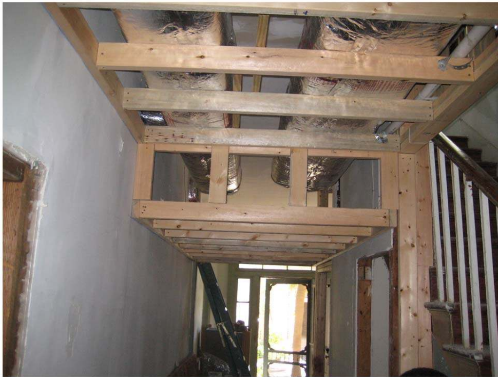
Supply and return in Hallway - Air Handler in Front Foyer ready to go in
